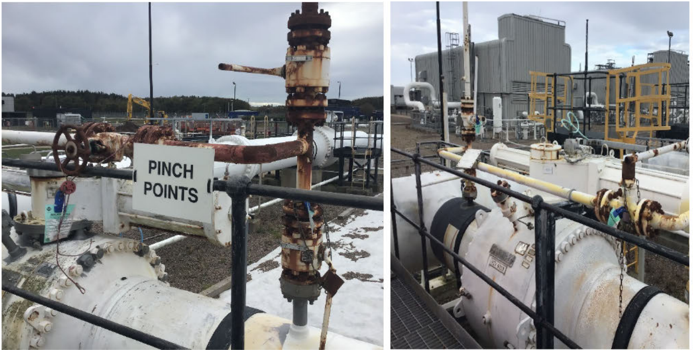
Figure 7 Category 6 corrosion defects on above ground pipework in the mixing area (located in area 6) of the terminal
